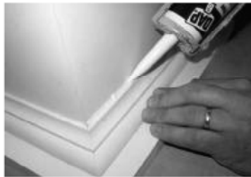
20) Caulk using latex caulking compound to fill an gaps & nail or screw holes.
