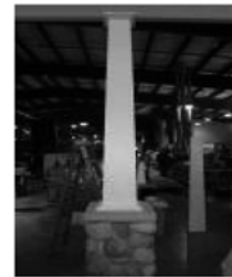
21) Clean surface of column with cleaner recommended by the paint manufacturer. Paint with 2 coats of acrylic latex paint.
