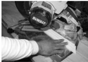
17) Using miter saw, cut base trim pieces to fit around bottom of column
